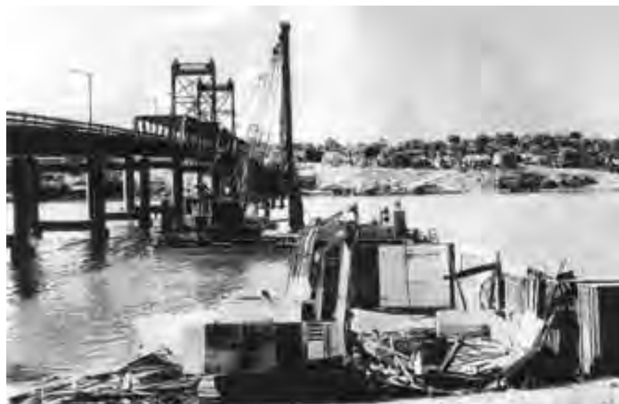
The old Clubhouse in the midst of demolition. Photo from the Ryde Historical Society. Photo supplied by Ted Kendrick.
