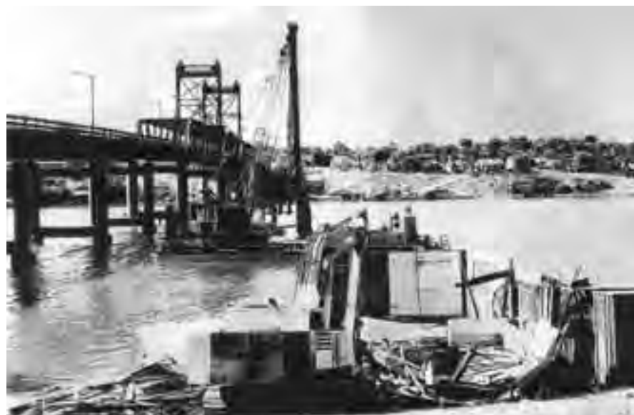
The old Clubhouse in the midst of demolition. Photo from the Ryde Historical Society. Photo supplied by Ted Kendrick.
